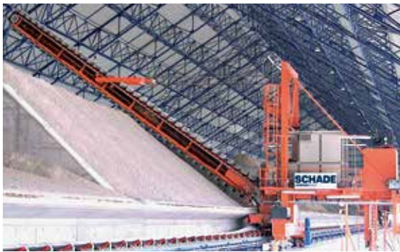
Cantilever Scraper Reclaimer, boom length 18 m, 200t/h, additives
