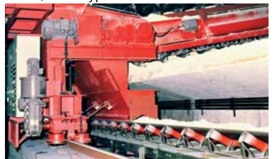
Direct discharge on belt conveyor
