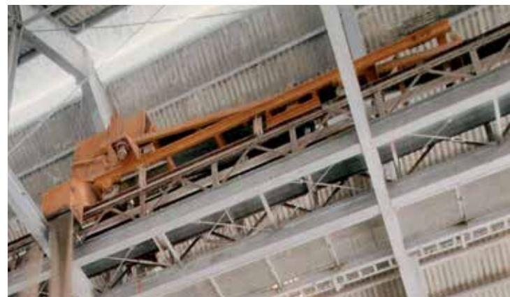
Fig. 5 Travelling tripper carriage
