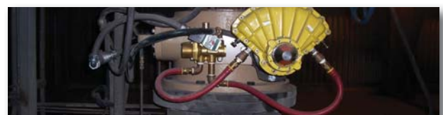
UCC TITAN HP Valve installed and in service with no failures for over 18 months. This valve has not required any maintenance since its original installation.
